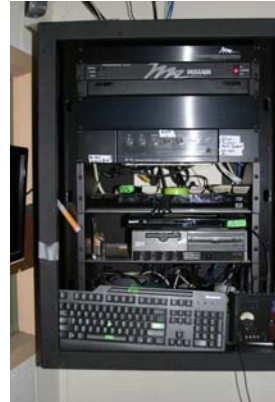
Middle Atlantic’s wall rack supports audio control and video distribution throughout the OSD’s Nightmare Factory Haunted House
